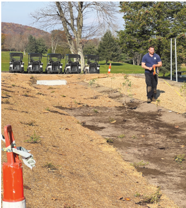
The Park and Recreation division of the Wolcott Public Works Department installed a Bio Retention Pond at the bottom of the Farmingbury Hills Golf Course parking lot recently. The purpose of the retention pond is to gather water runoff, filter it through the soil and vegetation, and eliminates the need for underground storm sewers.
