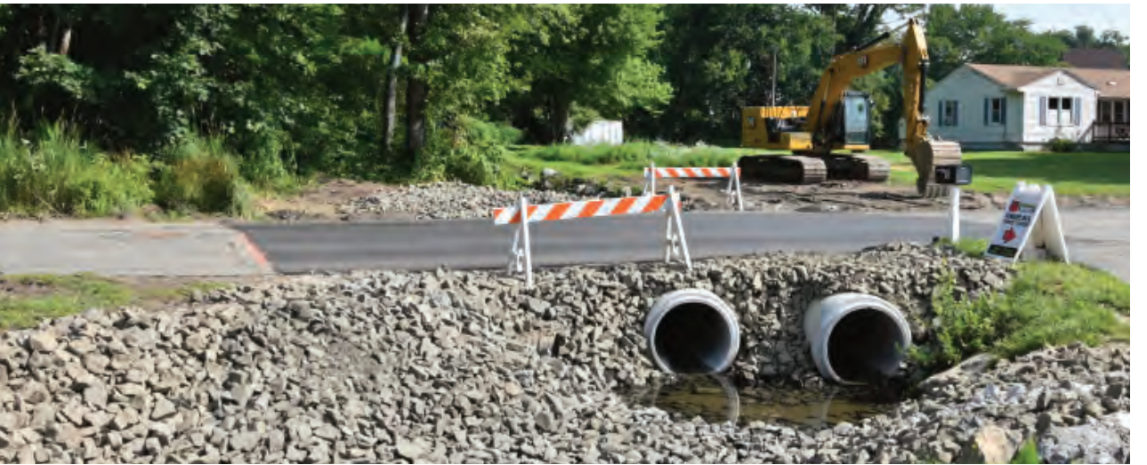
The Wolcott Public Works Department has been making repairs and upgrades at various locations in town that tend to flood during heavy rain downpours. This location on Longmeadow Drive near Wolcott Road had two large concrete pipes installed to handle such rain events and hopefully reduce or eliminate future flooding issues to local businesses.
