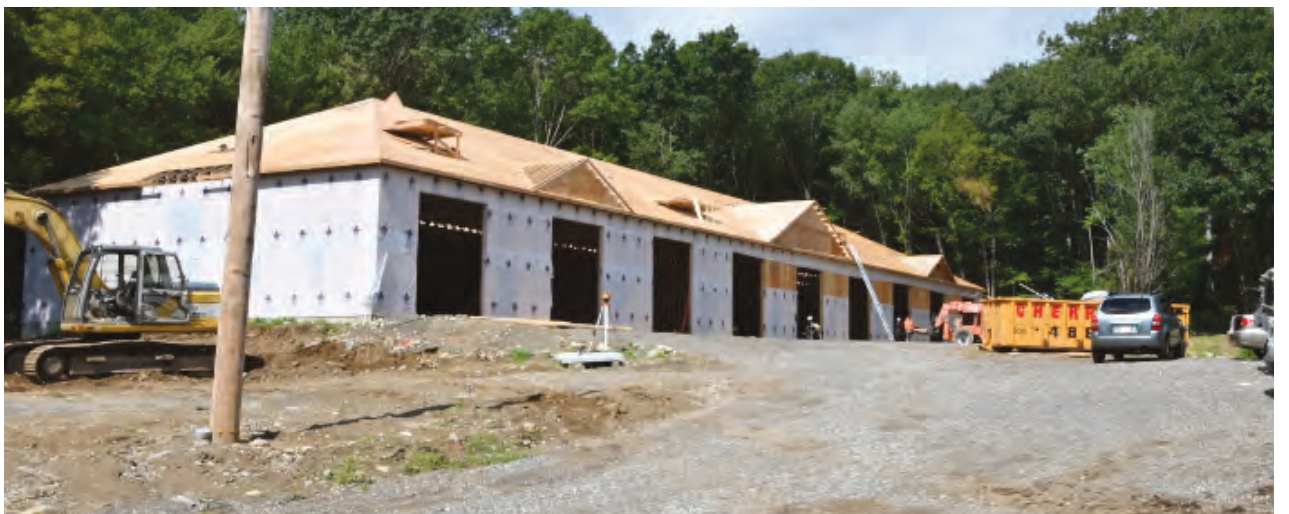
A new commercial building that can be subdivided for various commercial businesses is being constructed at 239 Wolcott Road. Research indicated there is a need for this type of building for businesses to utilize to store materials or vehicles or serve as office space to run businesses out of.
