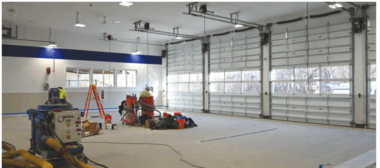
The new home for the Wolcott Volunteer Ambulance Assoc. is nearing completion. This photo shows a portion of the four bay garage nearing completion of work being performed. Chief William Barratt is hoping for an end of January 2025 occupancy. An open house dedication will probably take place in April.
