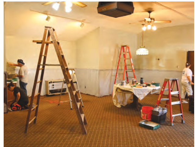
The Wolcott VFW Post on Wolcott Road is undergoing some renovation work thanks to a grant they received from Home Depot. Home Depot volunteers and contractors will be remodeling the meeting room in the lower level of the VFW hall and upgrading light fixtures and flooring during the course of the project.
