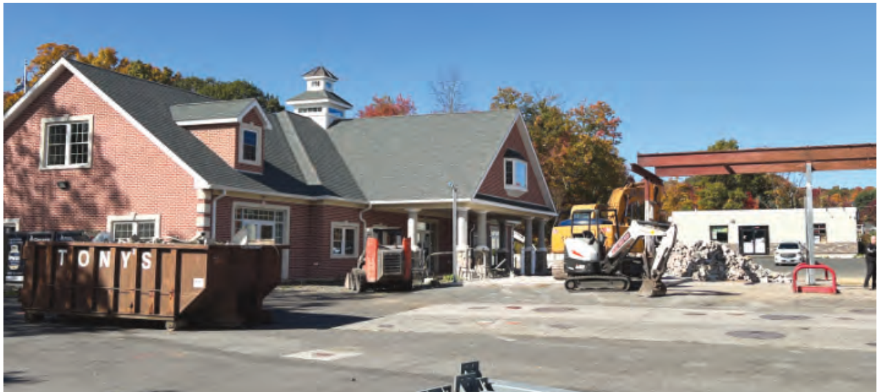
The new construction of Petro Pat's gas station on Wolcott Road continues with the removal of the old building and the gas pump island. A new island will be erected soon with new gas pumps and canopy.
