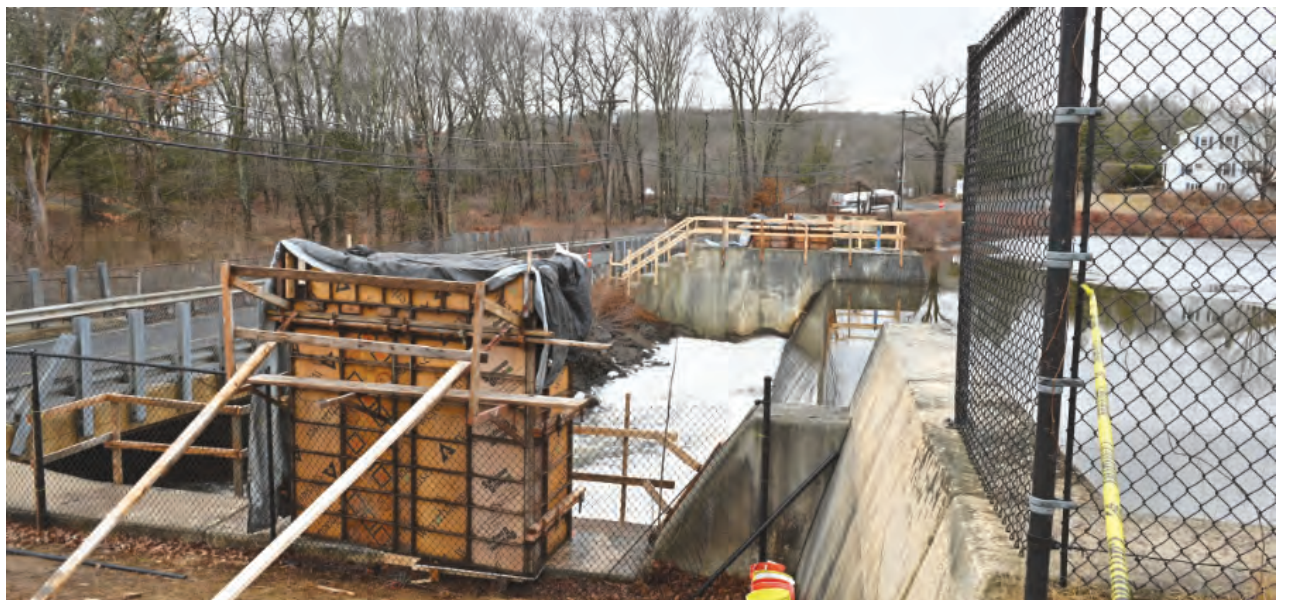
The process of putting a foot bridge over the lower dam at the Scovill Reservoir has begun. Construction workers were busy setting up concrete forms for piers that will support the new foot bridge. Once this part of the project is complete the new foot bridge will be delivered in sections and put into place on top of the piers. This bridge will eliminate the need of Mill Pond Way Trail users from having to cross Nichols Road in this area of the trail. Photography by Picard
